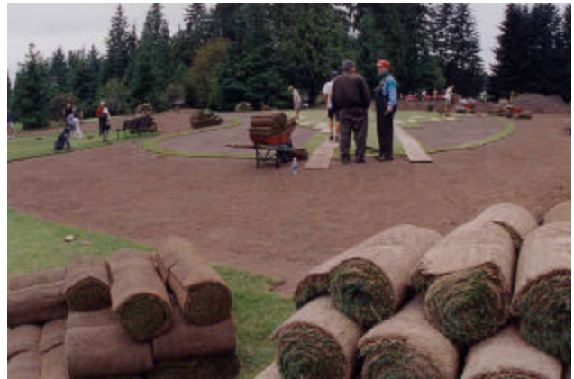
Renovations were underway at Capilano Golf and Country Club when we visited the green.
